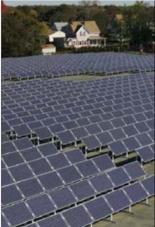
Brocton, MA PV installed following cleanup of former contaminated industrial site.
